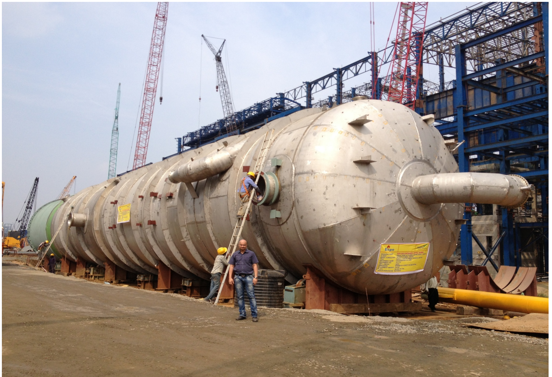
On the process of erection at Jindal Steel & Power Ltd. Angul Orissa INDIA Stripper Column (6.7 mtr. Dia; 46.26 mtr. Length, 260 MT. Weight). MOC SA 240 TP 316 L.
