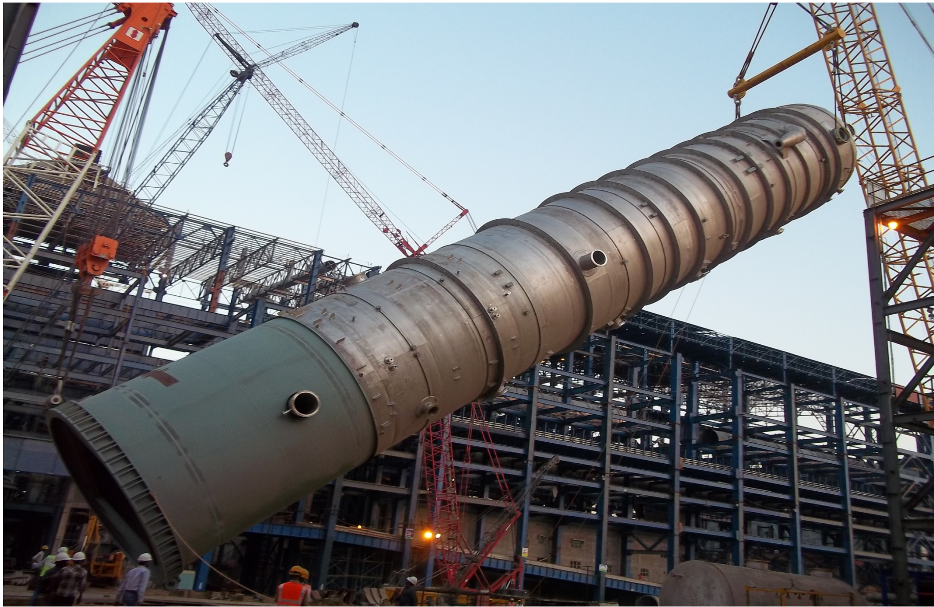
On the process of erection at Jindal Steel & Power Ltd. Angul Orissa INDIA Stripper Column (6.7 mtr. Dia; 46.26 mtr. Length, 260 MT. Weight). MOC SA 240 TP 316 L.
