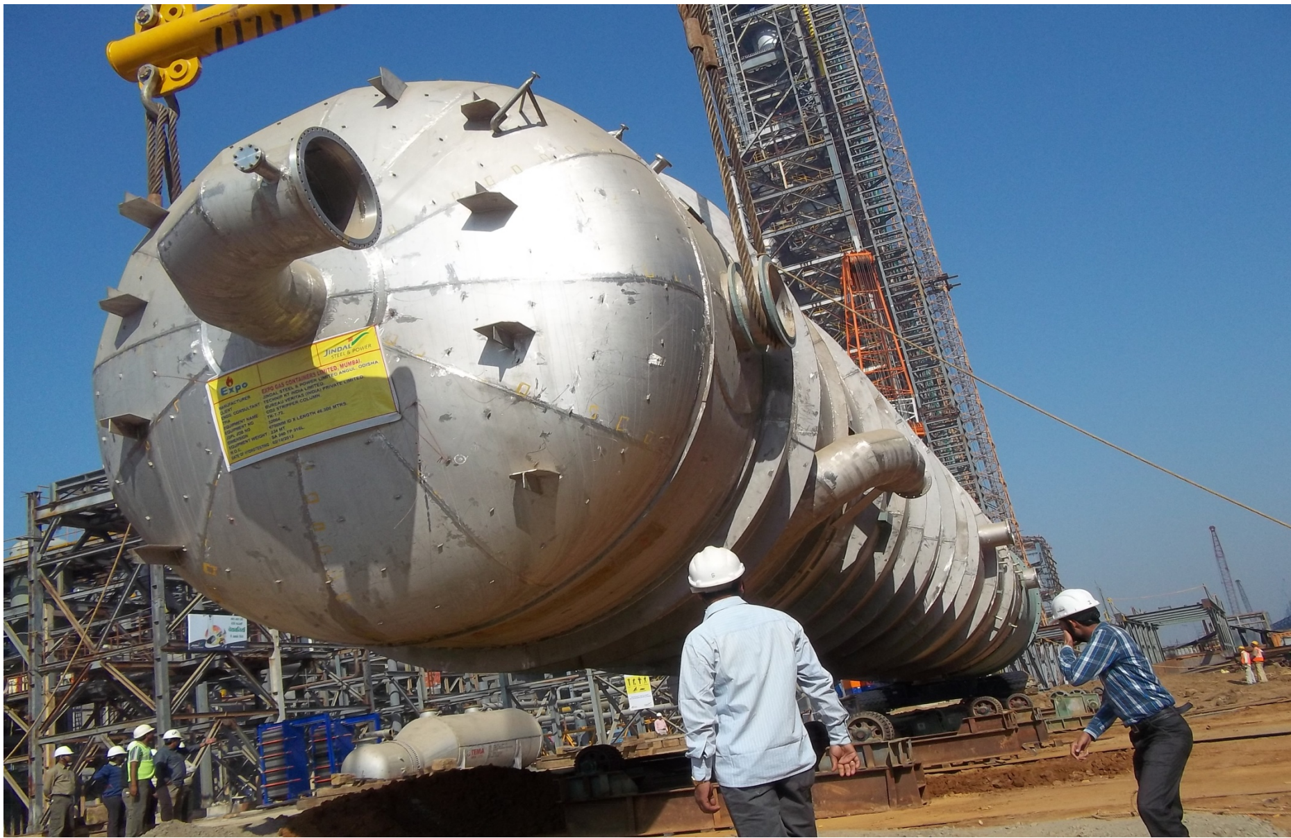
On the process of erection at site Absorber Column for Jindal Steel & Power Ltd, Angul Orissa INDIA (5.8mtr/ 4.6 mtr. Dia, 52.75 mtr. Length * 190 MT weight), MOC SA 516 Gr.70 & SA 240 TP 304 L
